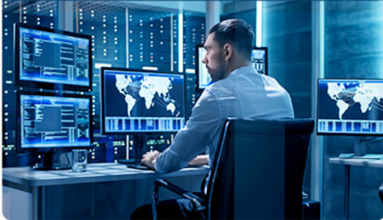
NOC (Network Operation Center)
